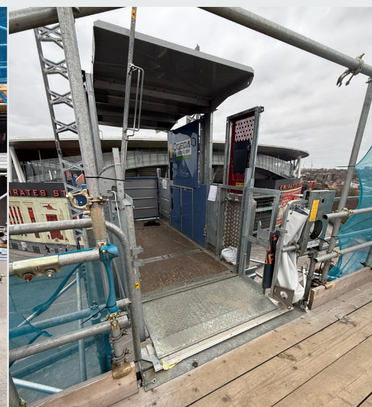
Hoist at landing position
