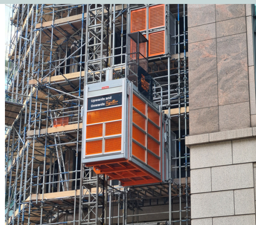
Hoist at the landing position showing Top Hat
